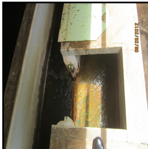
Figure 5: Flocculation Tank at Andankulam
