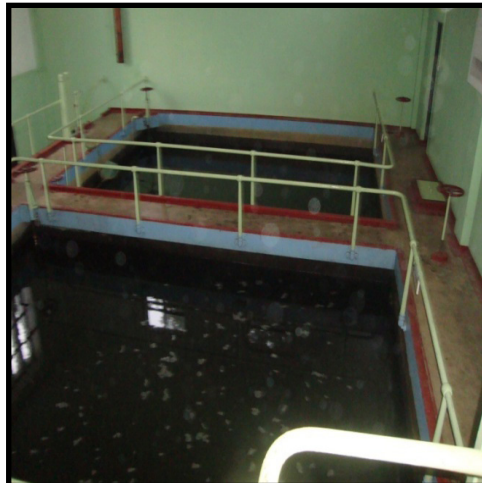
Figure 7: Filtration Tank at Andankulam
