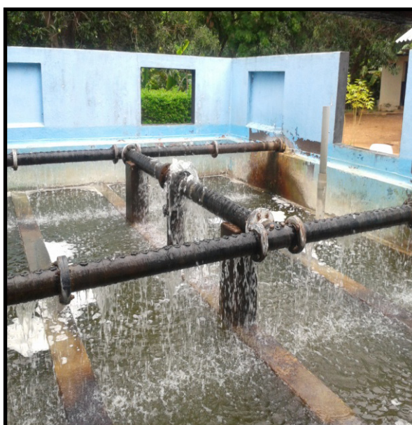
Figure 3: Aeration tank at Andankulam
