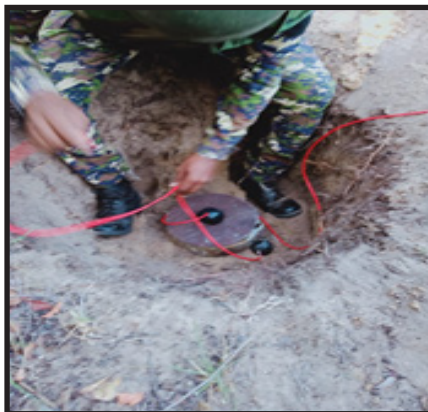
Figure 2: Preparing to Demolish an Anti-Tank Mine by SL Naval Personnel Source : Developed by the Author
