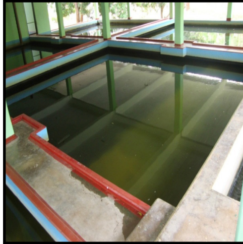
Figure 6: Sedimentation Tank at Andankulam
